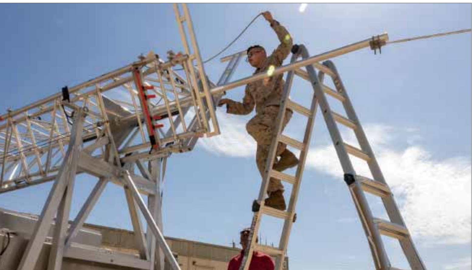
US Marine Corps Lance Cpl. Jesse Rushing, a transmission systems operator with Headquarters Battalion, Marine Air Ground Task Force Training Command, Marine Corps Air Ground Combat Center (MCAGCC) installs a 5G antenna for a 5G network demonstration. (US Marine Corps photo by Pfc. Ryan Kennelly)
