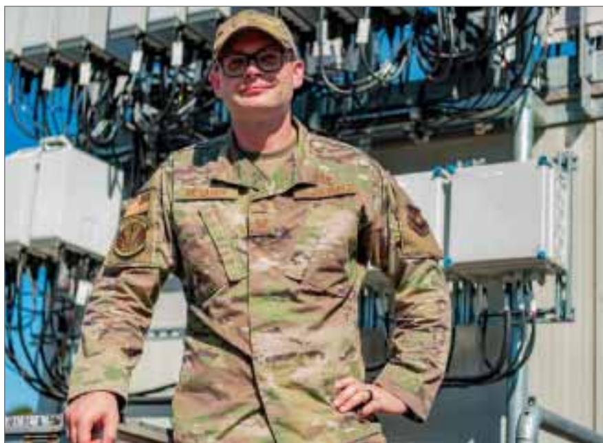
US Air Force Tech. Sgt. Ron Richards, 86th Communications Squadron non-commissioned officer in charge of cable operations, stands by a recently activated 5G cell tower at Ramstein Air Base, Germany. (US Air Force photo by Airman Jared Lovett)
